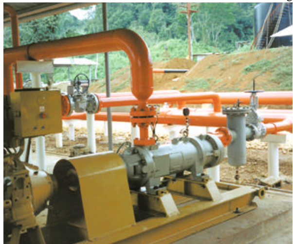
Figure 8 – Diesel Driven 3-Screw Pump at 1400 psi
