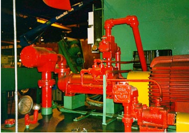
Figure 8 Hydraulic Pump With Right Angle Inlet Strainer
