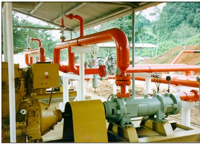
Figure 7 Diesel Engine Driver 100 Bar Crude Oil Pipeline Screw Pump in Guatemala, Central America
