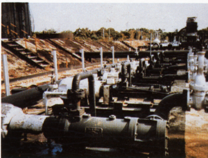
8L-640 Pumping Station - Indonesia
